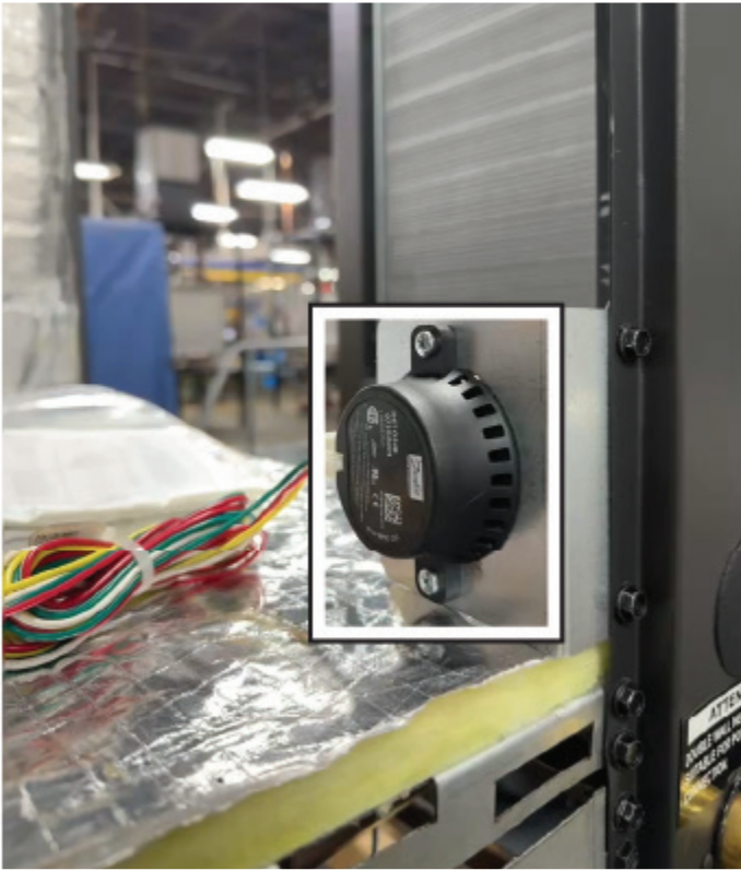
Figure 44: Vertical Blower Compartment Sensor
